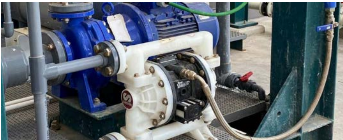
IMAGE 2: AODD pump in use at a sodium hypochlorite chemical factory
