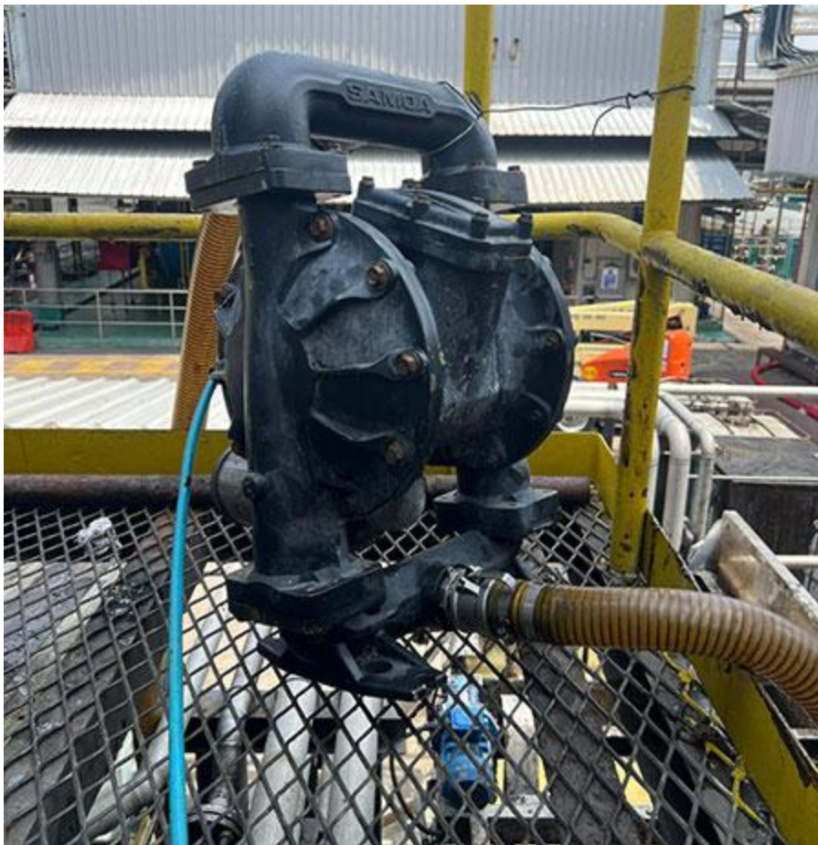
IMAGE 3: AODD pump for wastewater treatment plant
